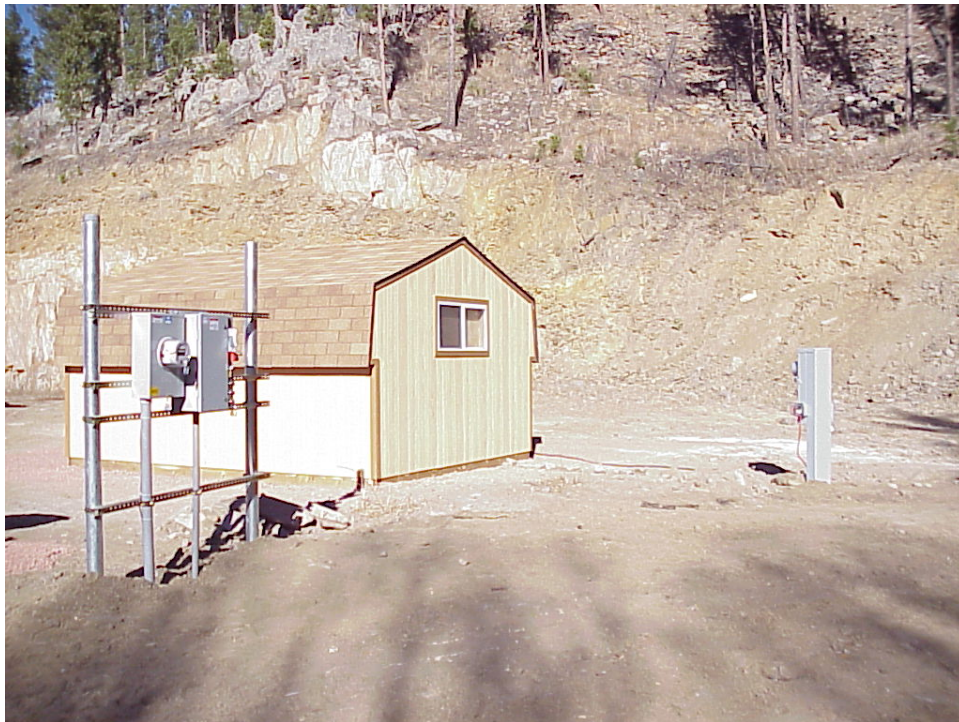
Figure 3. Keystone City Well No. 4.
