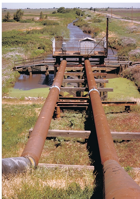
Pumps, such as these on Twitchell Island, remove agricultural drainage while maintaining the water table at a level low enough to sustain agriculture.
