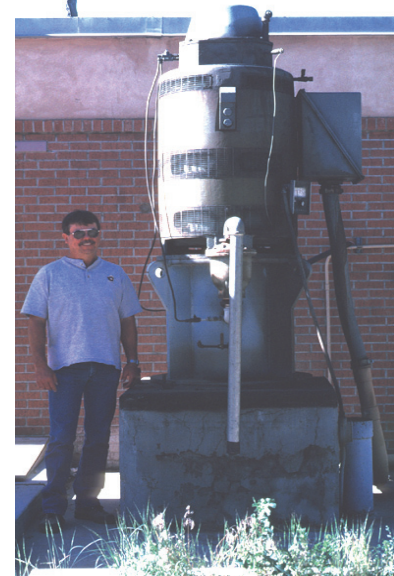
City of Albuquerque production well Leyendecker no. 1.
